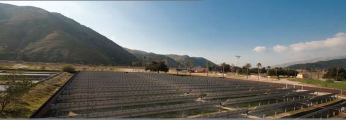
Harrah's Rincon Casino Photovoltaic Project Valley Center, California
